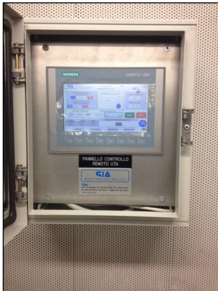
Figura 3-Comandi da pannello touch remoto in Control Room
